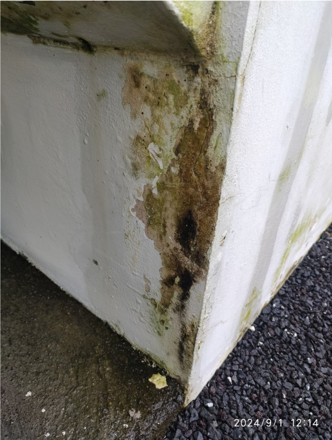
CRACKED, MOLDING, AND UNSEALED, ONE YEAR OLD
