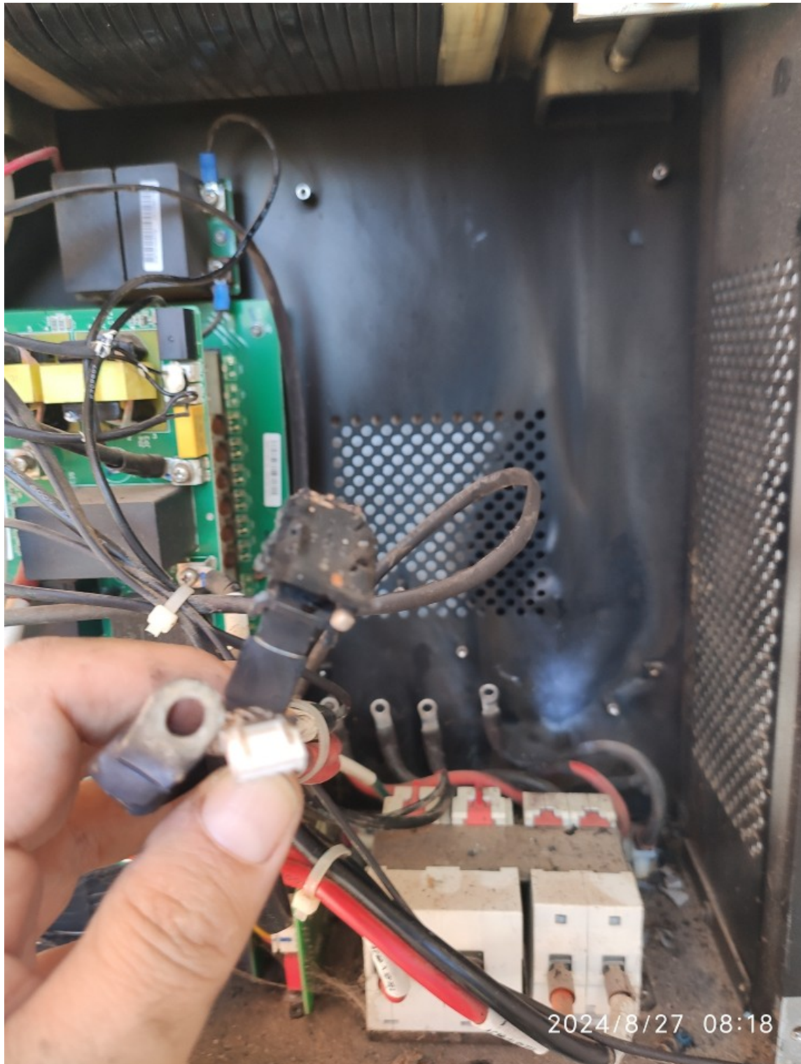
IMAGE 2 OF INVERTER / FIRE
