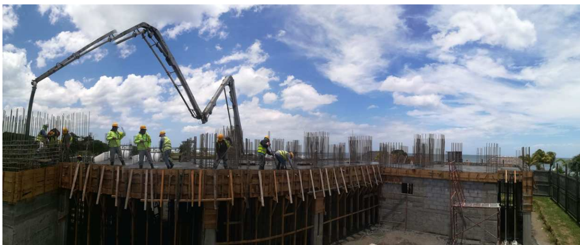
The first building of 12 condominiums is under construction with completion expected Q4 2020.
